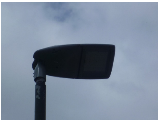
Figure 3.3 – shows a close up of one of the LED street lights shown in figures 3.1 and 3.2.
