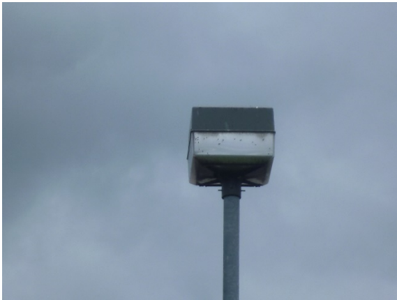
Figure 3.6 – shows a close up of one of the column mounted luminaires shown in figures 3.1 and 3.2.
