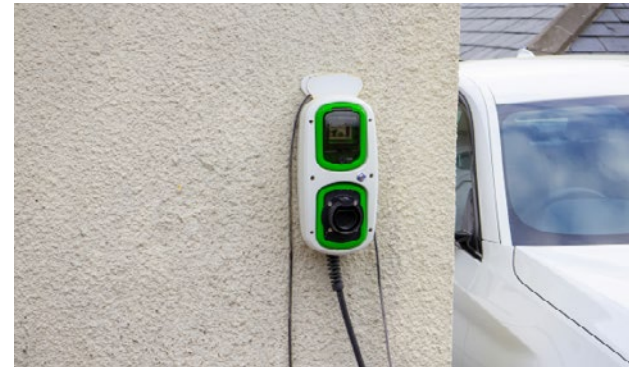
Figure 55: Electric charging points should be located discretely, where possible avoiding building façades visible from the road or public pathways to retain the character of the building.
